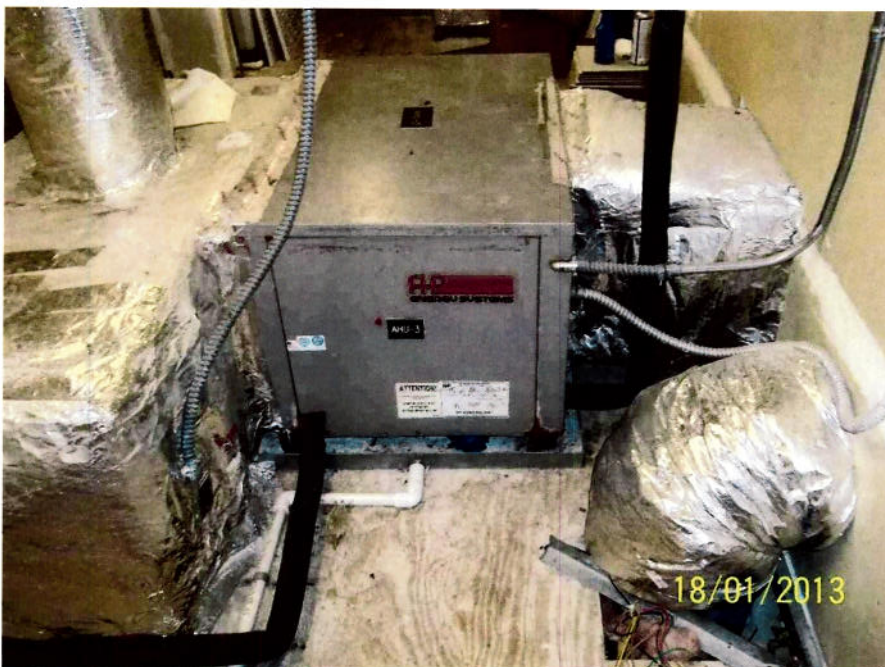
AHU-3: Located above 2nd floor bathrooms. Remove and dispose of properly. Replace and full reconnect with new unit.
