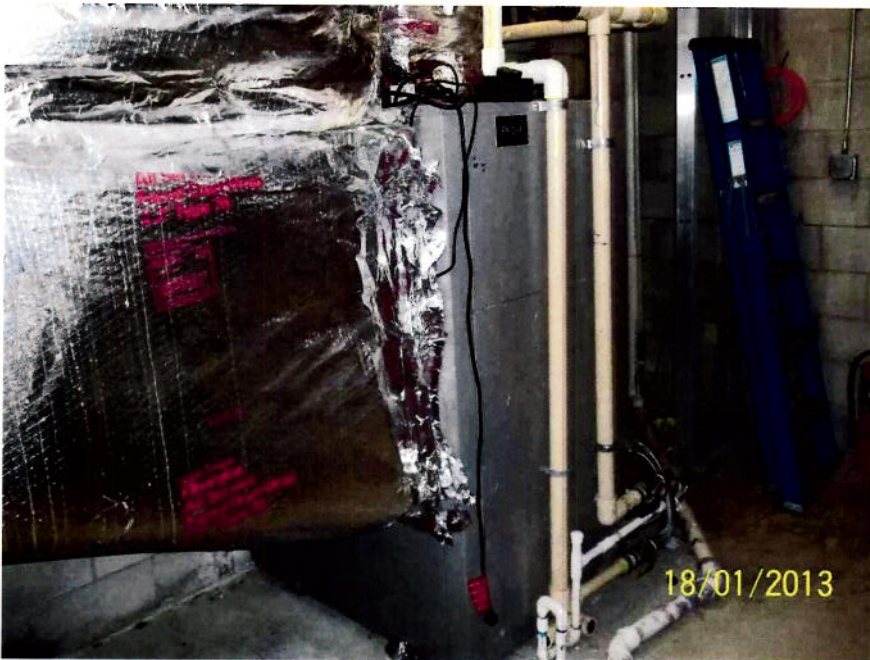
Package Unit#1: Air intake duct needs reworked/replaced and supported properly to allow proper filter installation and replacement for new unit.
