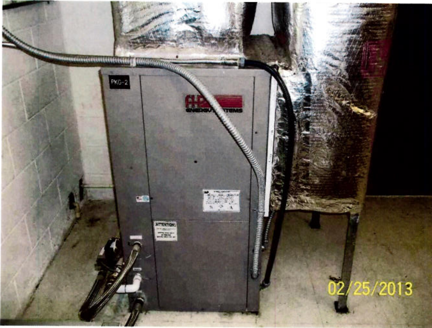
Package Unit #2: Located in storage room off Training Room. Full replacement. Dispose of old unit properly.
