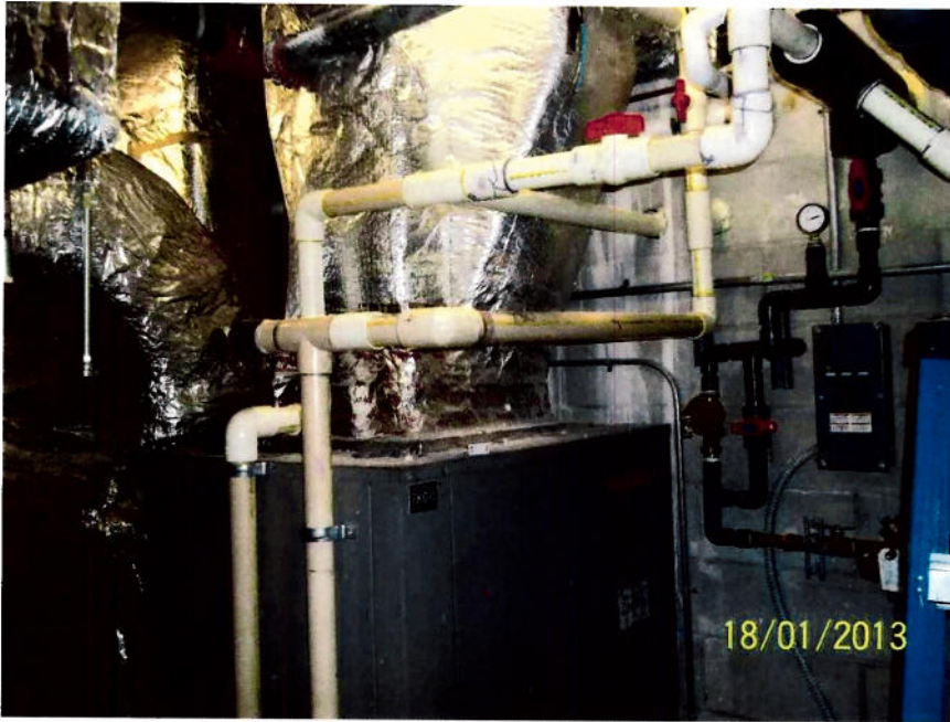
Package Unit#1: Re-circulated water coolant piping and discharge duct.
