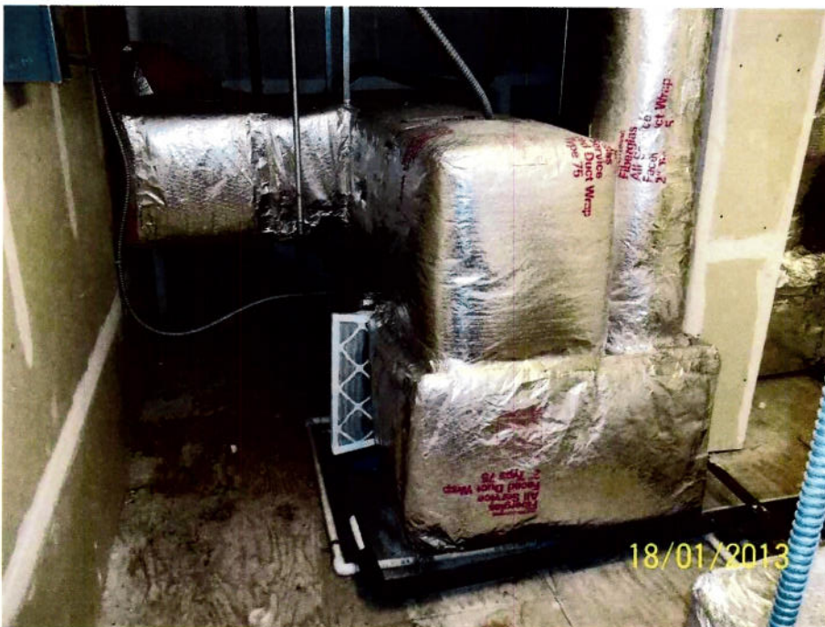
AHU-4: Located above 2nd floor bathrooms. Remove & properly dispose of unit. Replace and full reconnect with new unit.
