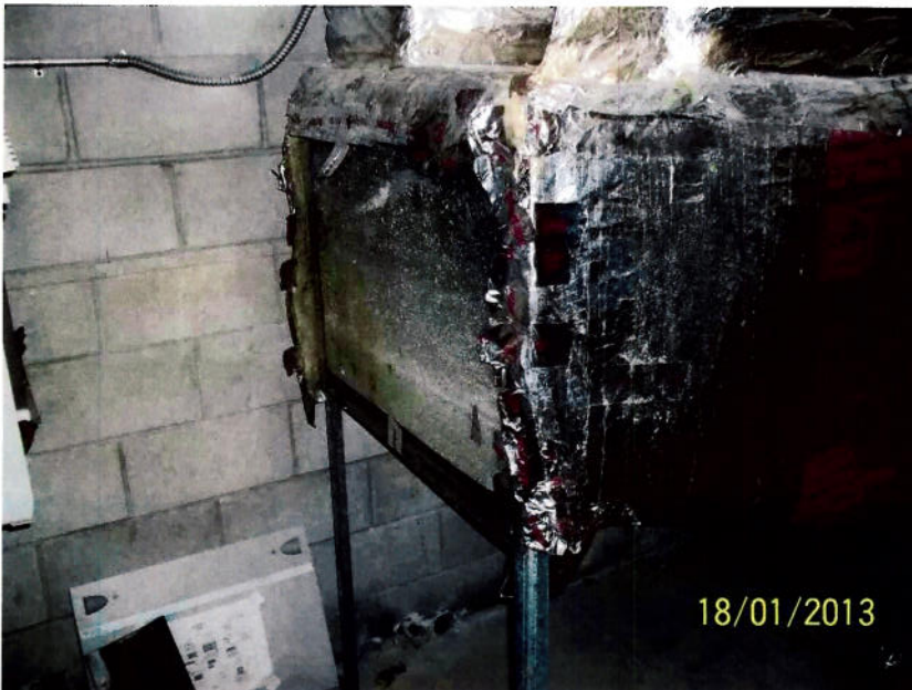
Package Unit#1: Air intake duct needs repair/replacement. Make-shift filter and plexiglass needs removed and duct repaired/replaced.
